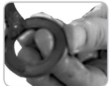
Figure 14.10. Greasing the bearing covers
